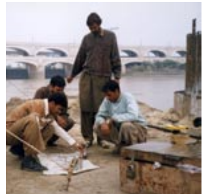
Execution of confirmatory borings at the bridge piers. A newly constructed pile at the right and the upstream Sukkur Barrage in the background.
