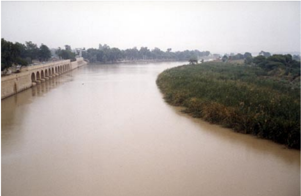
Upstream irrigation channel weir (left). Artificial island (right) which developed in the early years of operation as a result of excessive siltation at bays 6-10.
